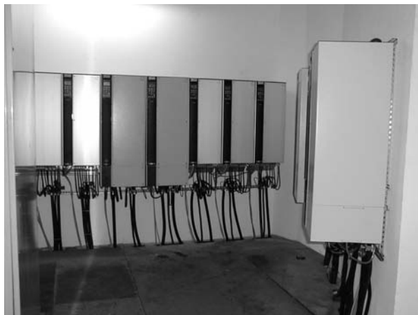
Slika 7. Frekventni pretvarači smešteni na zid elektro sale Figure 7. The frequency converter placed on the wall of the electro installation room
