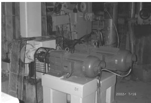
Slika 6. Pogonski motori i reduktori partije premaza karton mašine Figure 6. The drive motor and inductors of the coating part of the drying unit
